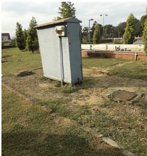
T EARTHING PITS
