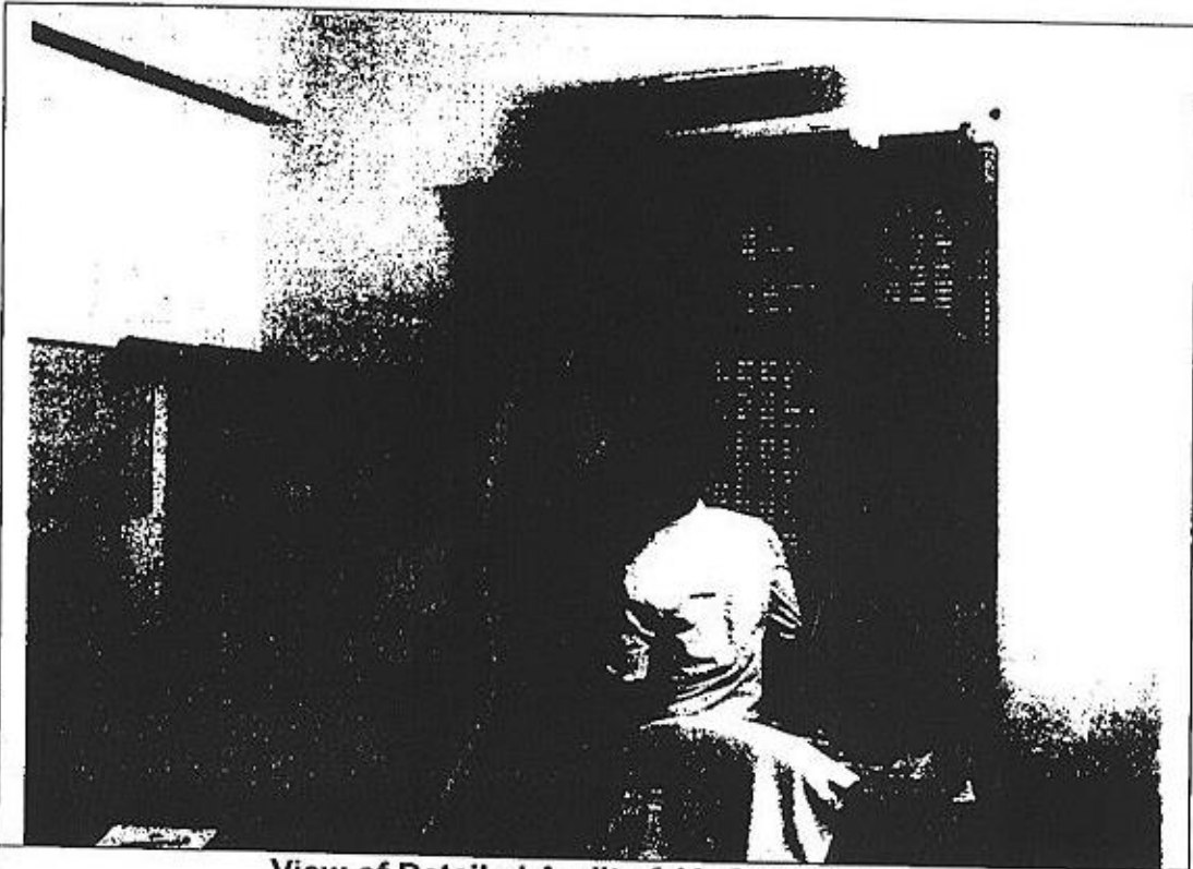
View of Detailed Audit of Air Conditioner
