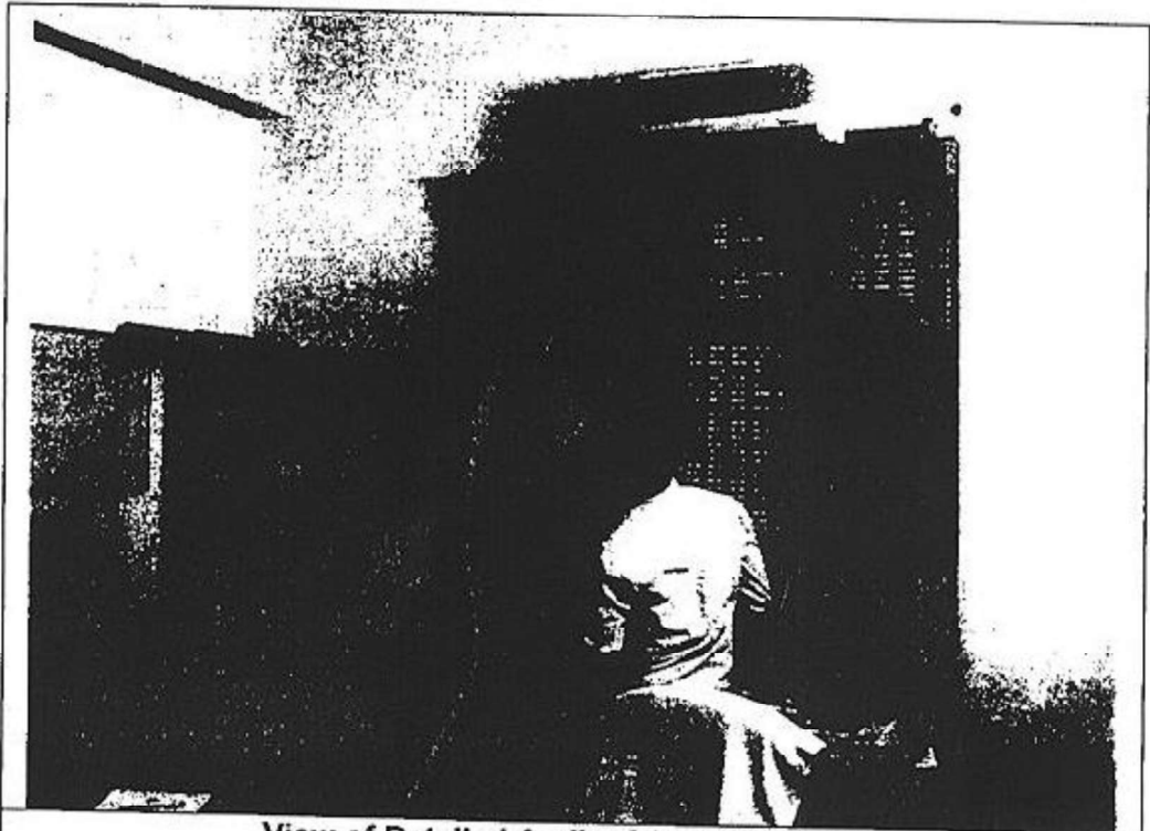
View of Detailed Audit of Air Conditioner
